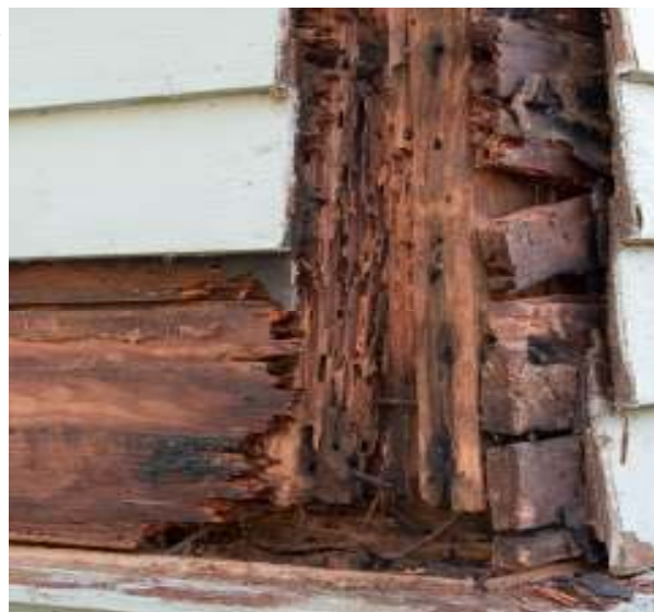
Figure 3: A wooden house frame damaged by termites. Termites harbor cellulose degrading bacteria in their digestive systems that allows the termites to use wood cellulose as an energy source. Cellulose comprises approximately 50% of the total biomass of wood.
